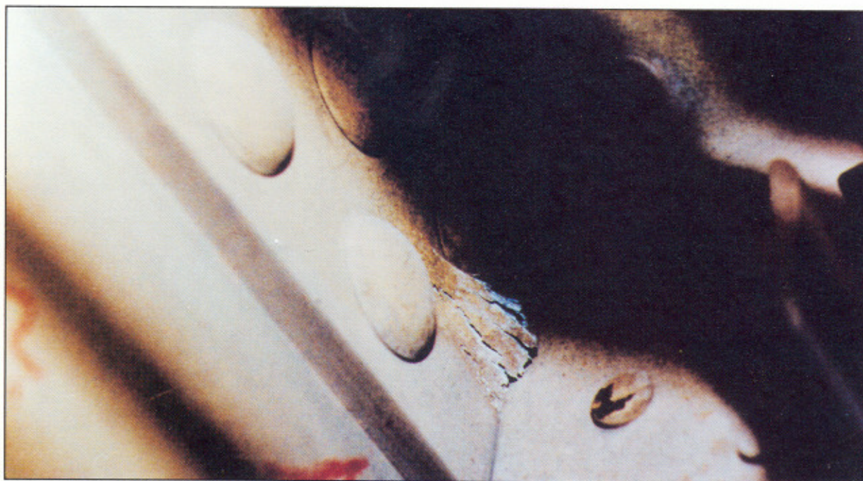
FIGURE 5-9. SPAR CHORD CORROSION
