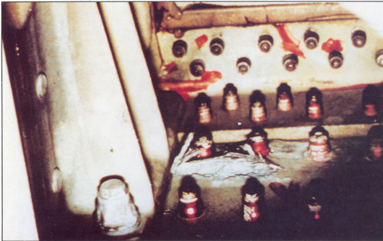
FIGURE 2-9. SEVERE EXFOLIATION CORROSION
